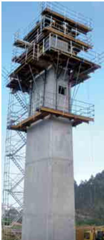
CR-250 brackets in pier execution with pouring, intermediate, main and cones recovery platforms. The access is provided by BRIO scaffolding ladder
